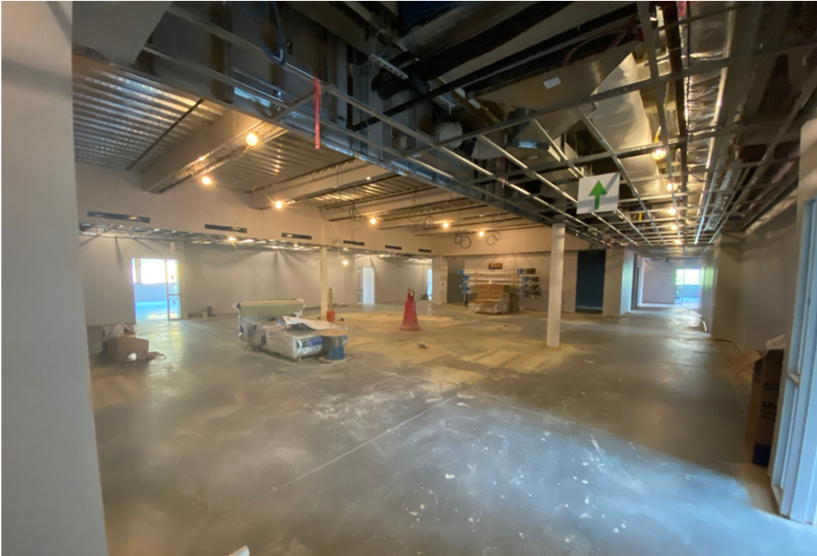
Construction Update Meeting | Walter P. Carter & Lois T. Murray Elementary School | August 12, 2020 www.baltimore21stcenturyschools.org
