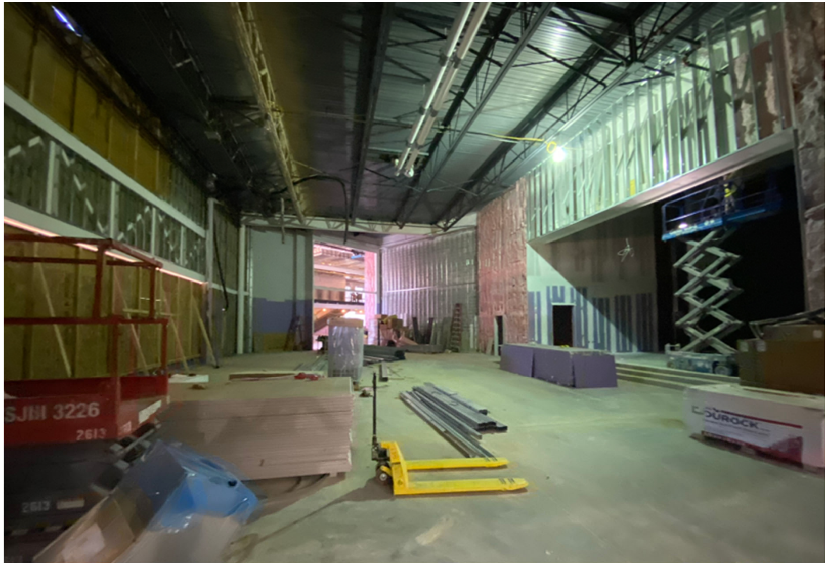
Construction Update Meeting | Walter P. Carter & Lois T. Murray Elementary School | August 12, 2020 www.baltimore21stcenturyschools.org
