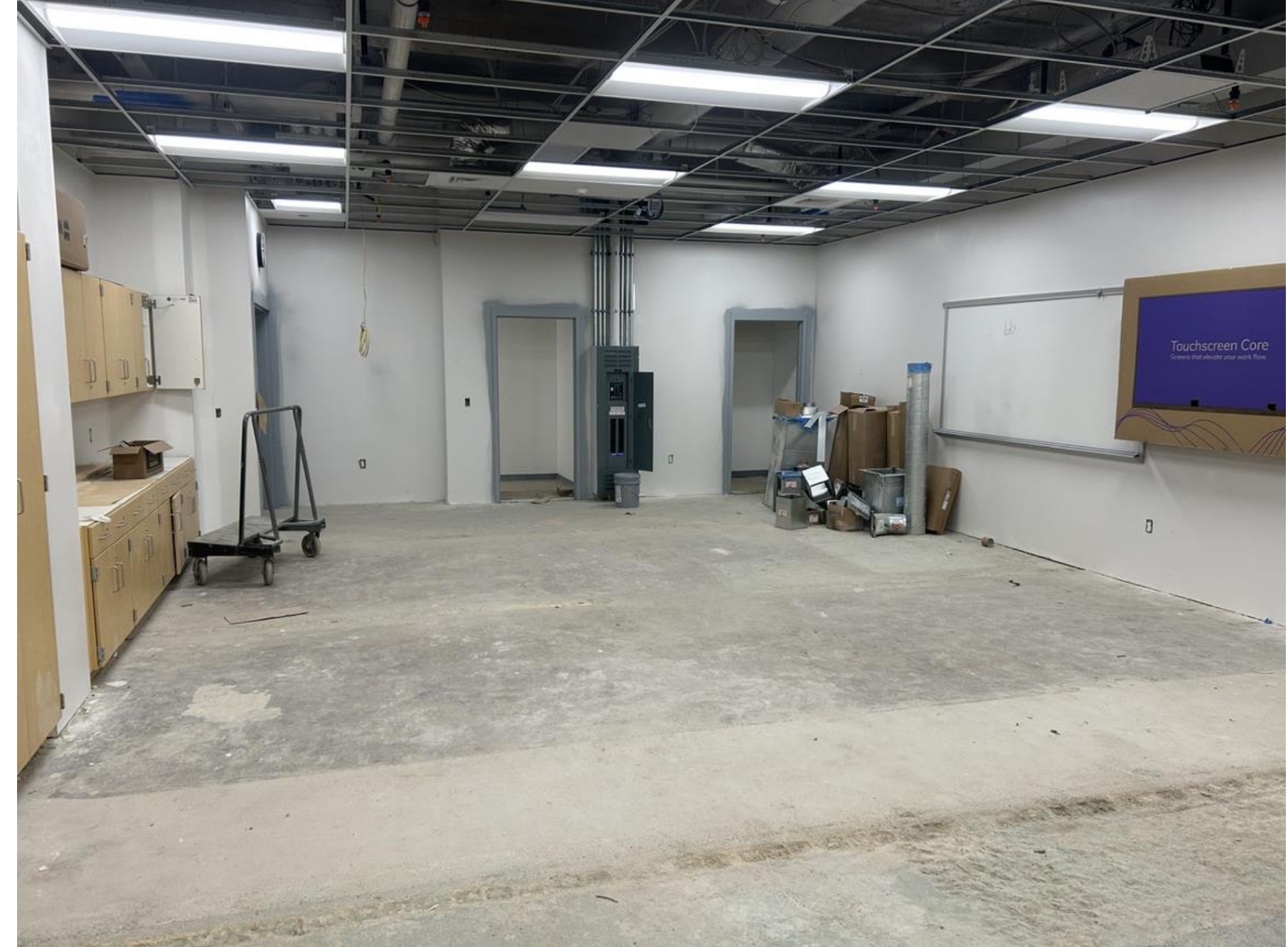
CONSTRUCTION ROOM – This is the classroom portion with finish ceilings being finalized & flooring to follow.
