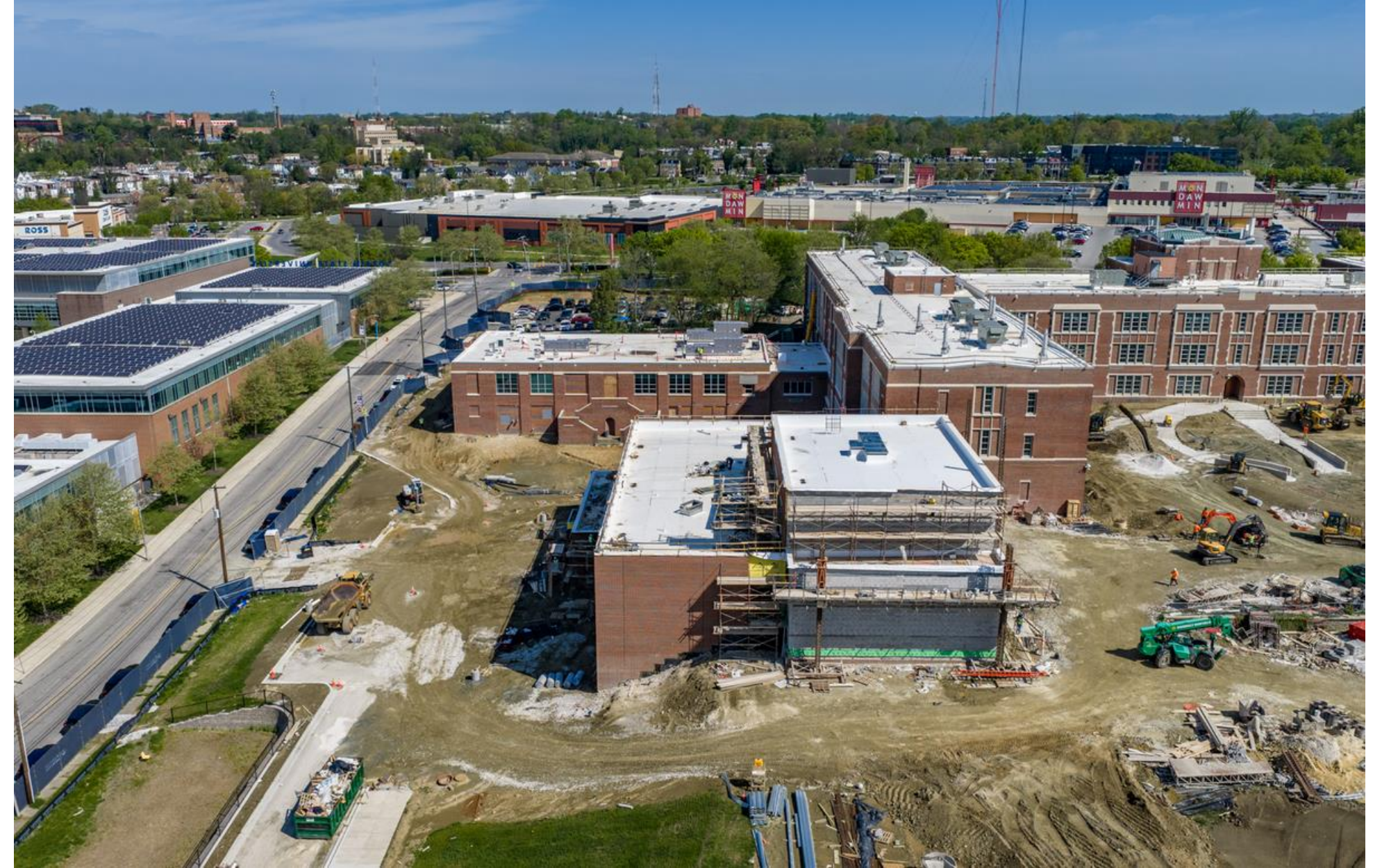
NOW – Briscoe Addition w/ Auxillary Gym is constructed & site concrete is progressing.
