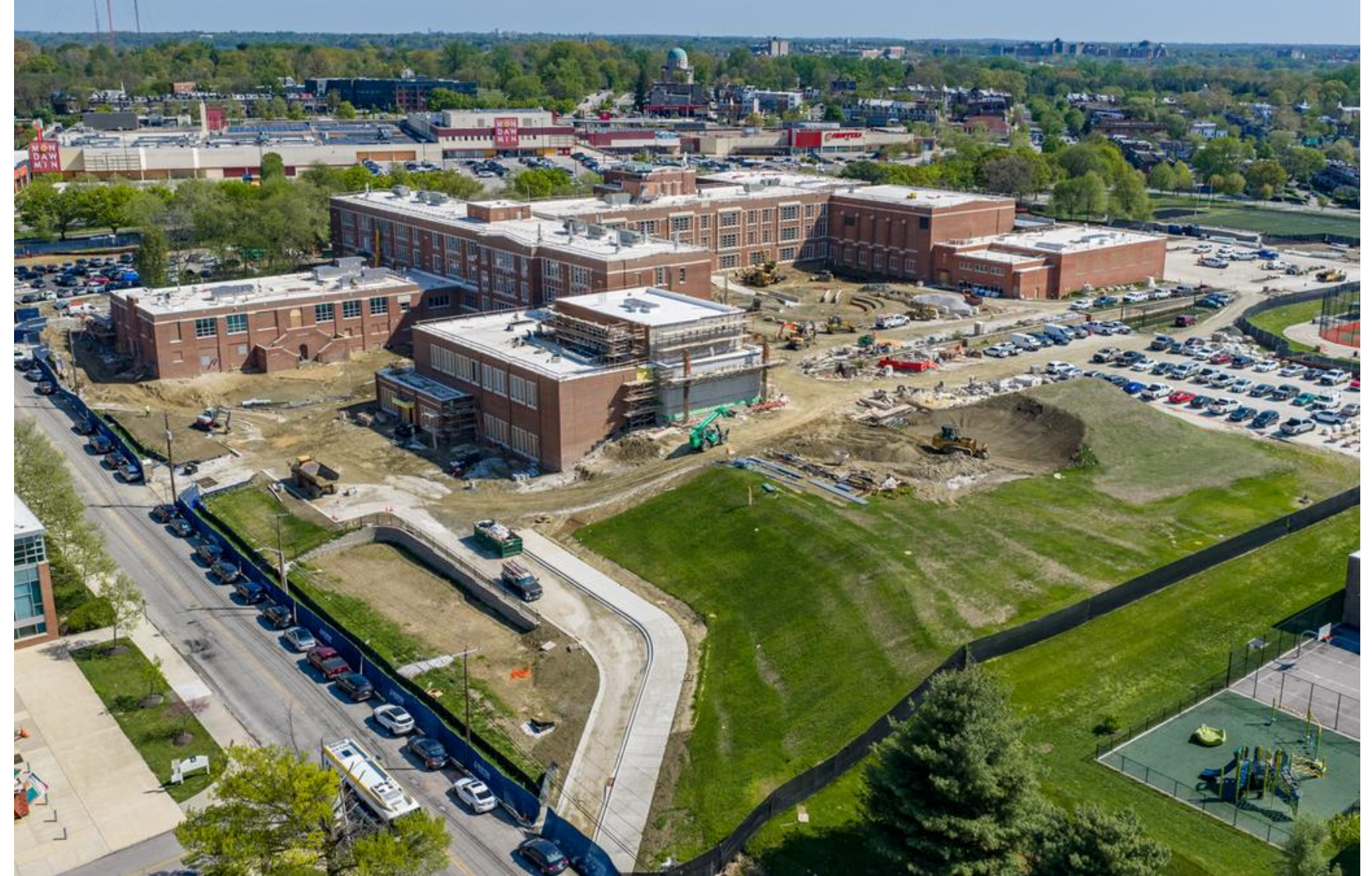
NOW - Briscoe Addition is in place, Student drop-off in progress & Douglass outdoor learning is progressing.
