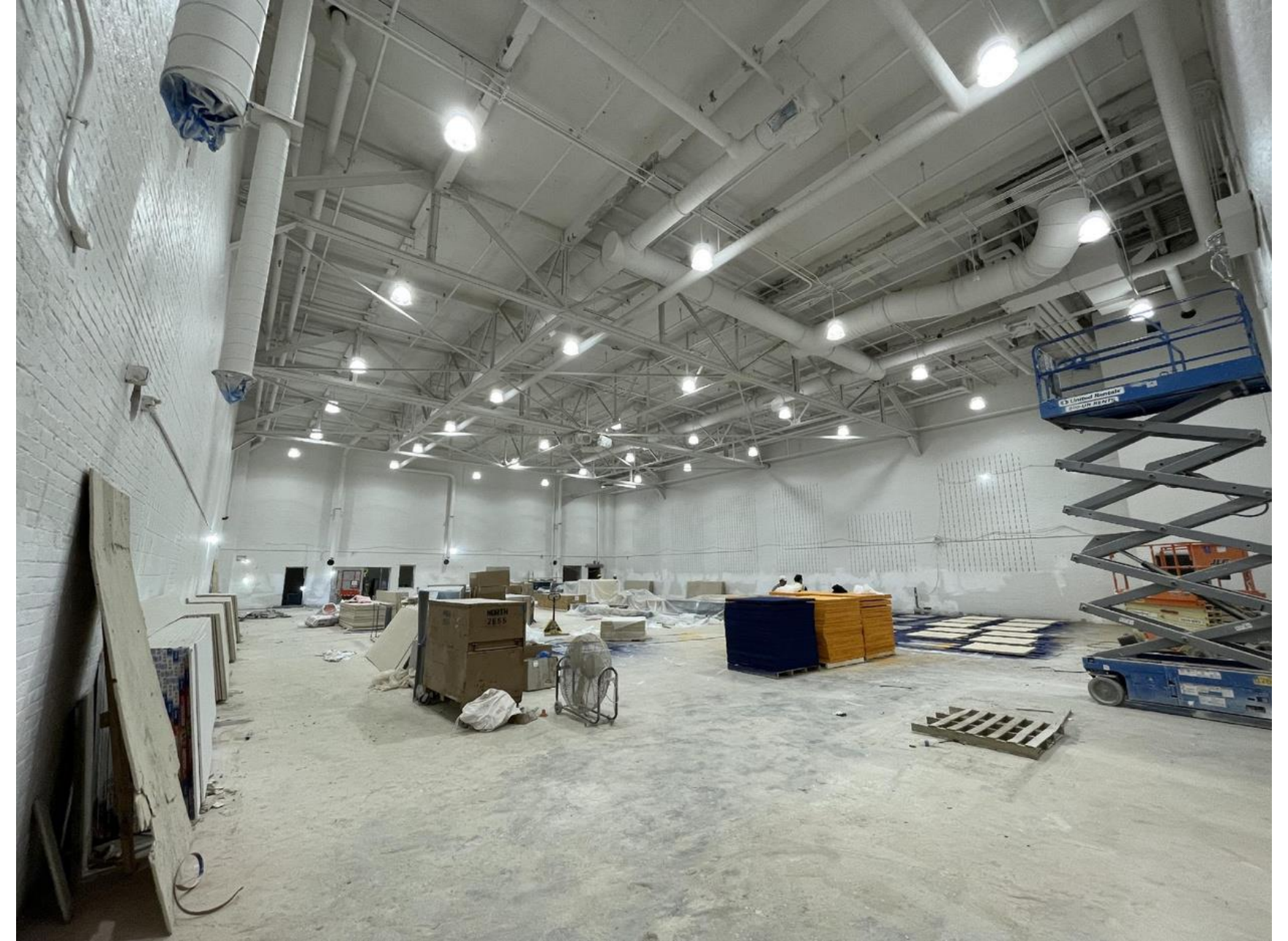
DOUGLASS GYM – Finish paint is complete, permanent lights are installed, sound panels are being prepared for installation, to be followed by Athletic equipment
