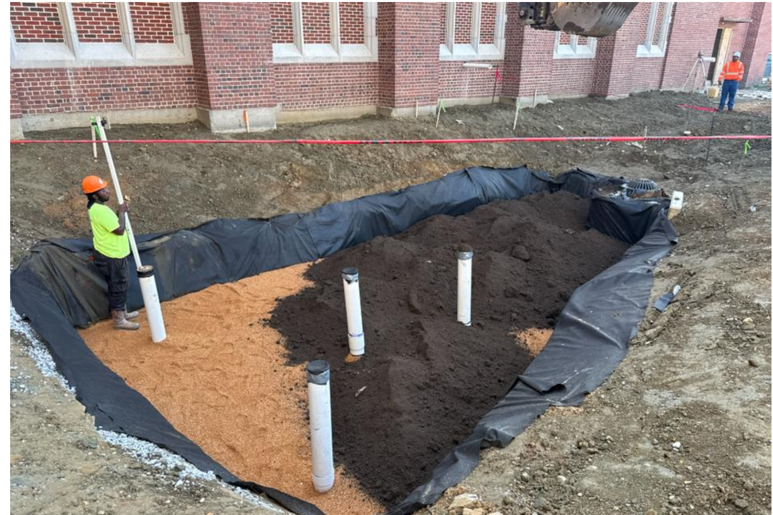
BIO-PONDS – currently being constructed with all utility work complete, stone base installed with filter media being placed, followed by plantings
