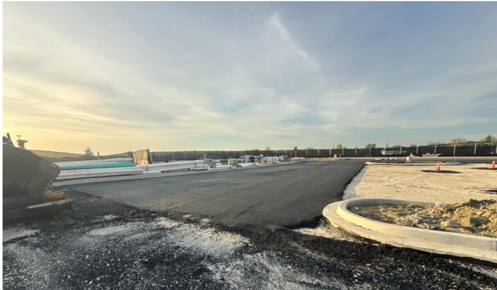
EAST PARKING LOT – parking islands have been completed, along with light pole bases & base paving has begun
