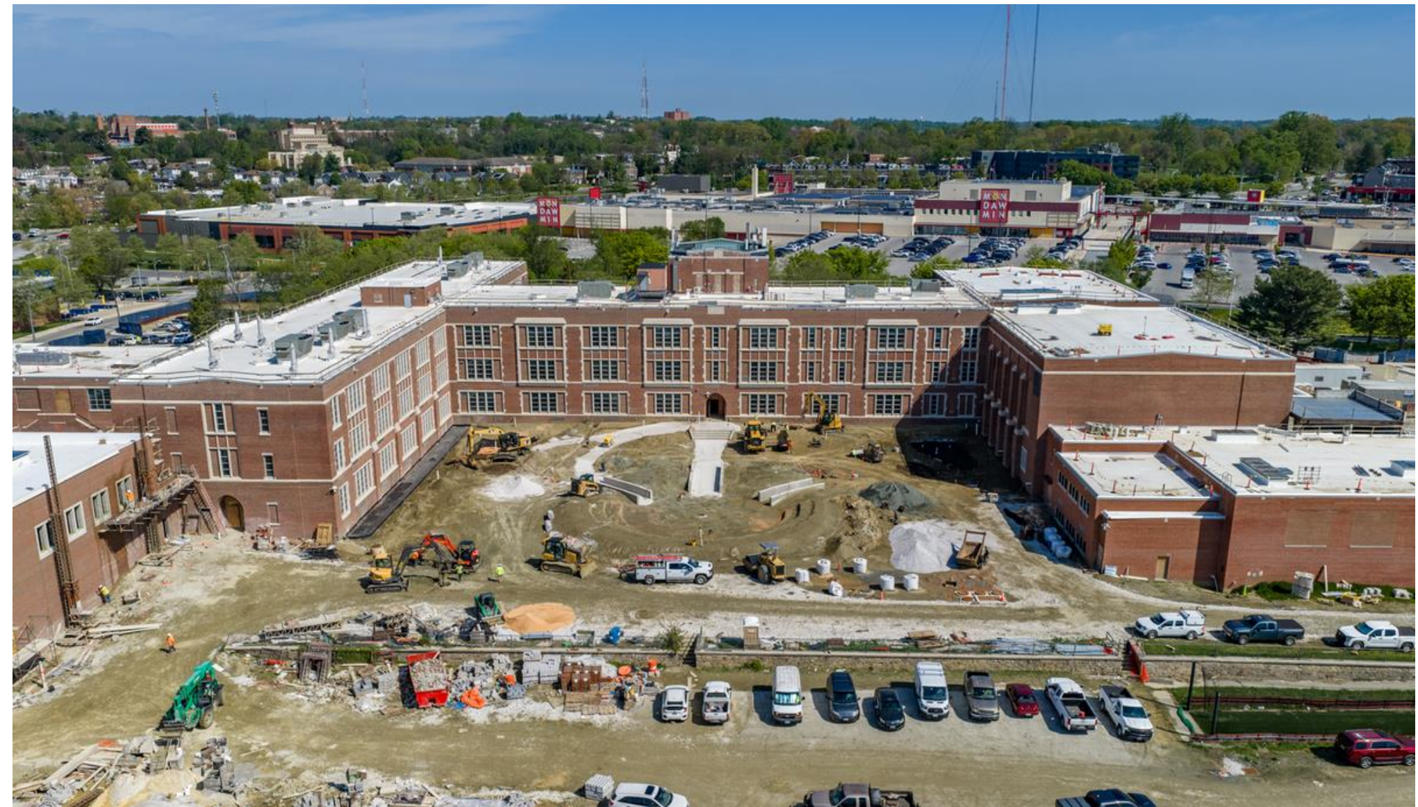
NOW – The new roof is substantially complete, windows have been installed, rooftop equipment setting has begun & outdoor learning has developed.
