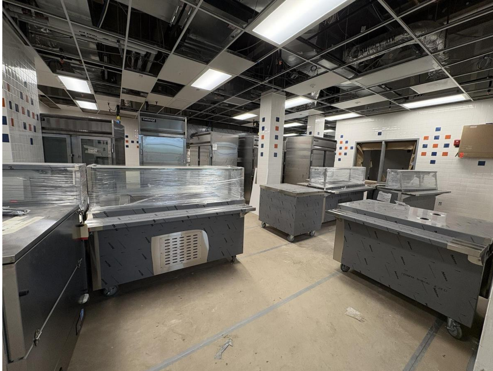
KITCHEN – Finished flooring & wall tile is complete, Walk-in's are constructed with all equipment being set for final connections
