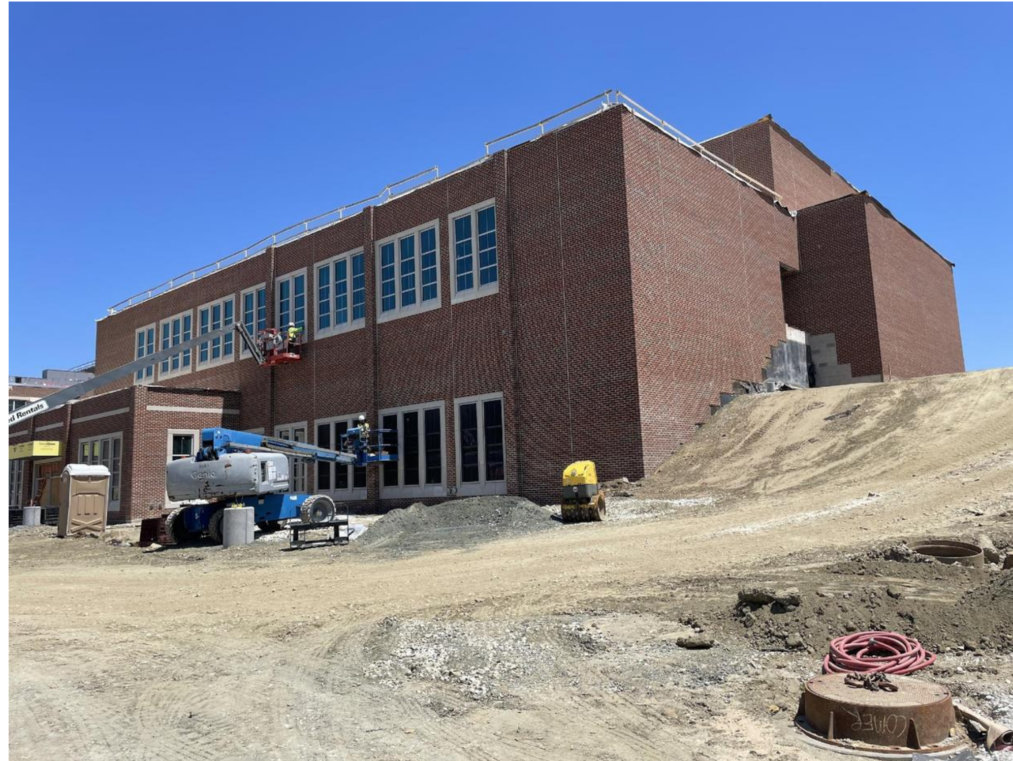
BRISCOE – exterior walls are finished with window installation concluding with caulking & the security screen installation
